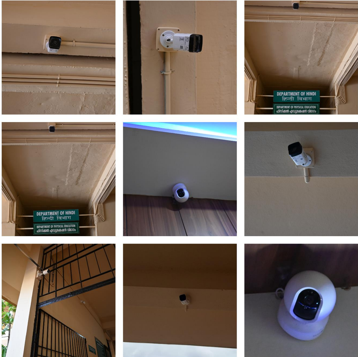
Image 18: CCTV installed at various locations of the campus
